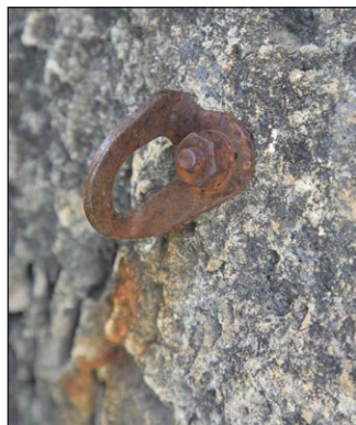
A rusty bolt - probably sound but difficult to trust
